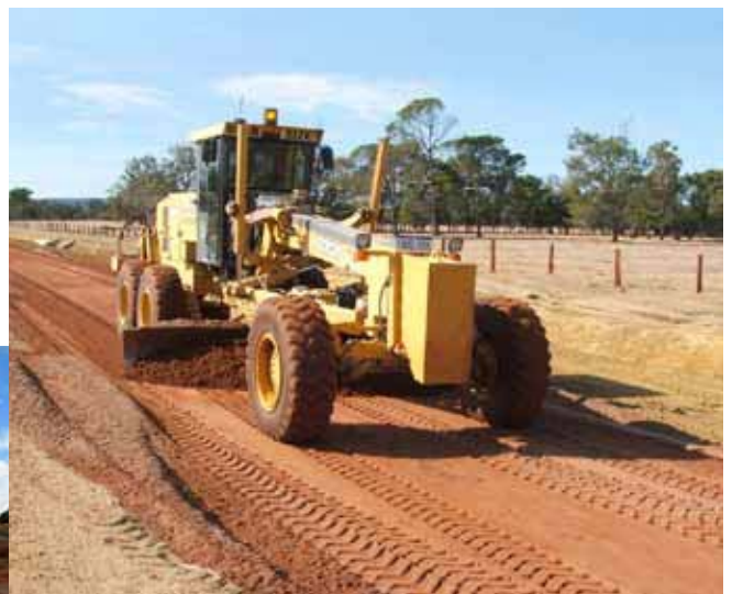
Grading of sand recovered from bauxite residue in the construction of a section of Greenlands Road. Image courtesy of CSRP.
