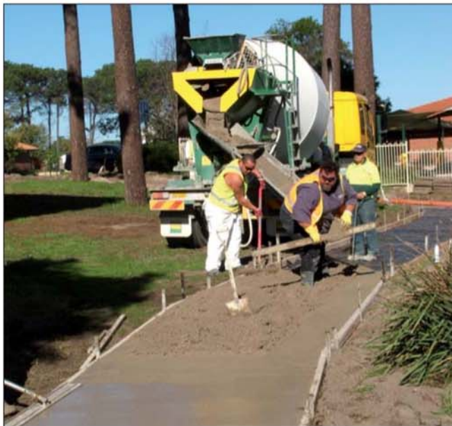
Figure 6 Fly ash geopolymer footpath being laid at Curtin University in 2008. (photo courtesy of CSRP).
