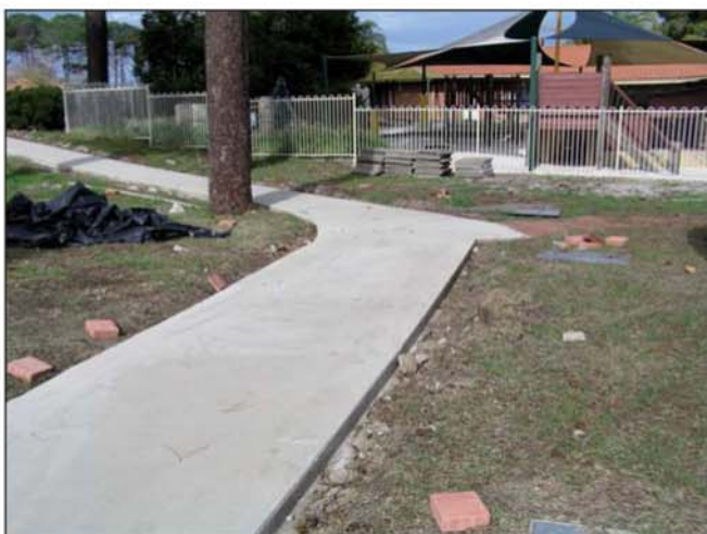
Figure 7 Completed fly ash geopolymer footpath at Curtin University in 2008. (photo courtesy of CSRP)
