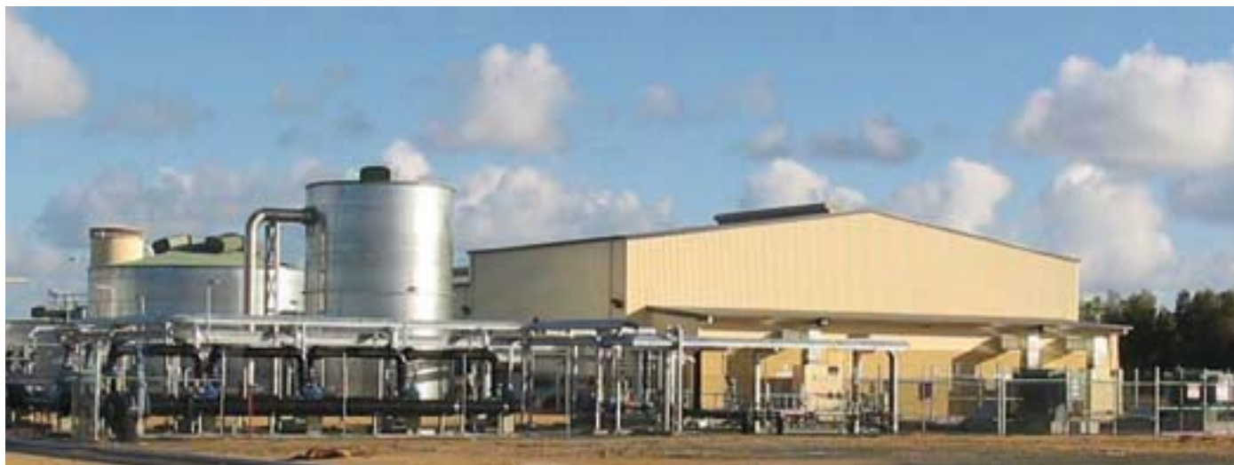
Major water saving: This water reclamation plant at Kwinana has reduced the use of scheme water by six gegalitres per day since its commissioning in 2004.
